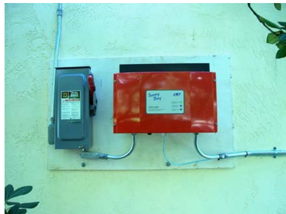
DC PV array cut-off switch and inverter.
