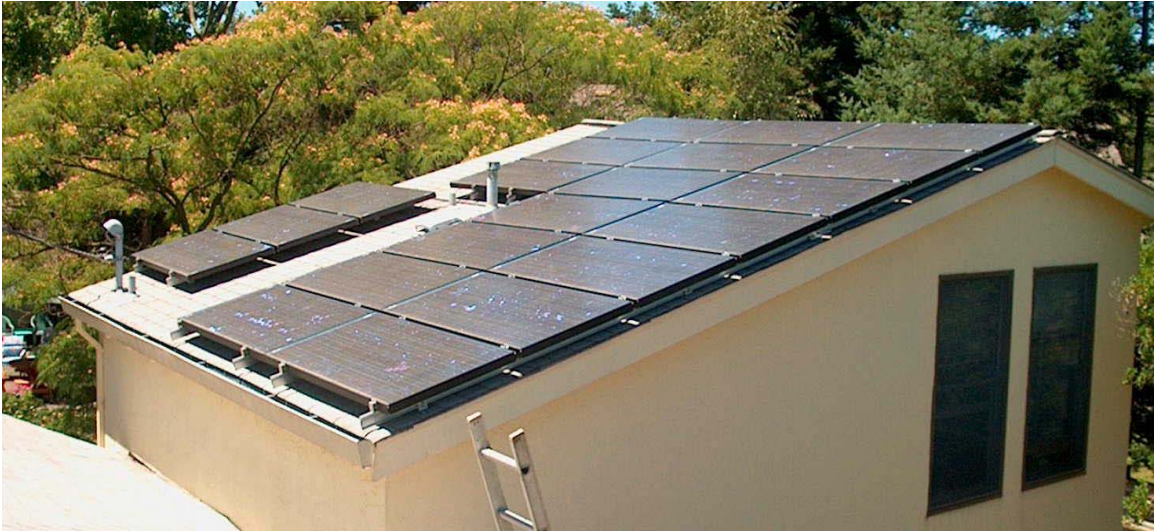
Twenty installed panels facing south (note N. roof access to clean gutters).
