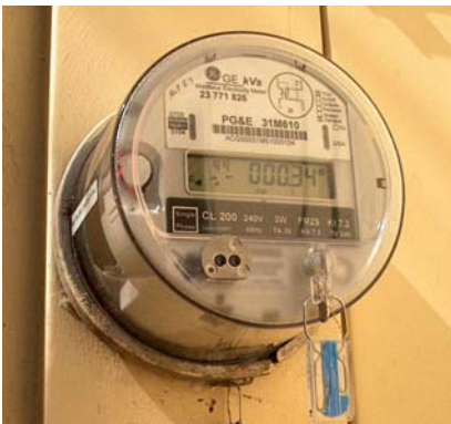
A new digital Time-of-Use Meter was installed.
